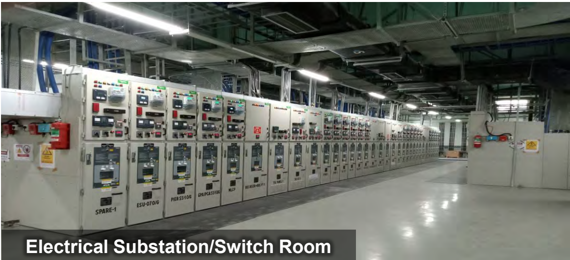
66/11 Kv GIS Substation
